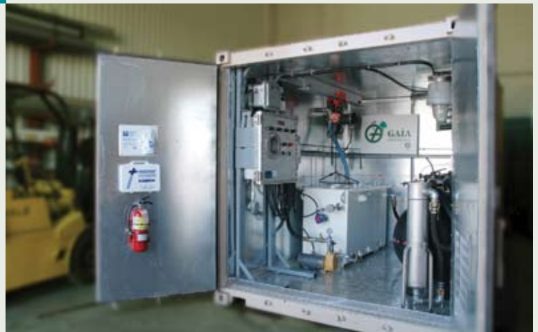
Process Room – multi-phase extraction system
